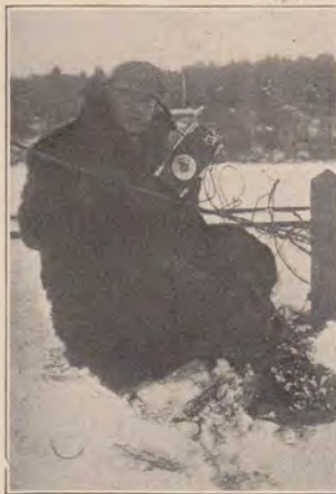
LINE FOREMAN CHISHOLM Testing out line on Toll Section 143 near Littleton, N. H.
