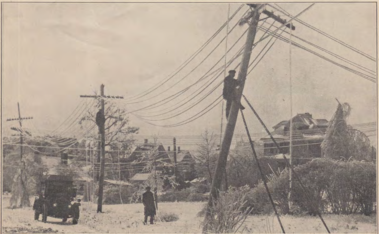
"SERVICE FIRST" Plant men at work restoring service on broken lines between Stoneham and Woburn. In snow, sleet and rain our slogan "Service First" helped Plant men "carry on."
