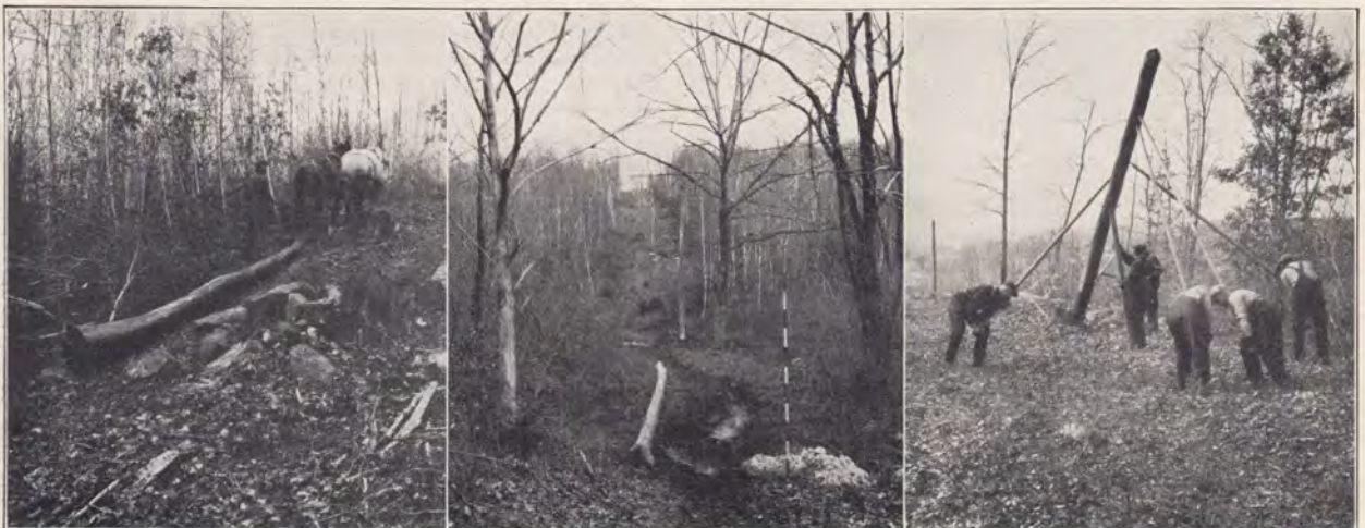
BUILDING THE APPONAUG—VALLEY TOLL LINE WHICH WILL CARRY PROVIDENCE—VALLEY AND EAST GREENWICH—VALLEY TRUNKS
