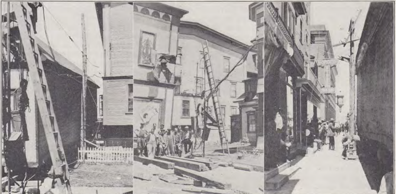
WHEN A BUILDING GOES ON A JOURNEY, THE TELEPHONE EQUIPMENT MUST GO ALONG TOO
