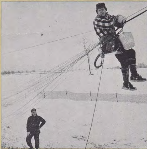
Gardner Hopwood, Manager in Alburg, Vt., for the Home Telephone Co., Inc., works on cable repair in Alburg.
