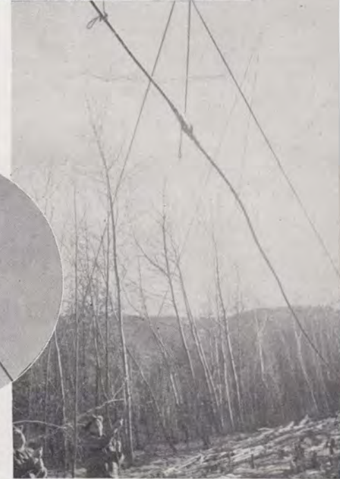
Above: After ground splicing the cable is carefully raised preparatory to lashing.
