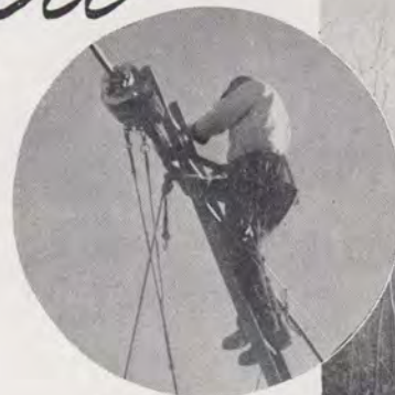
Above: The cable lasher "bug" approaches splice. It is then moved to other side of splice to finish lashing.
