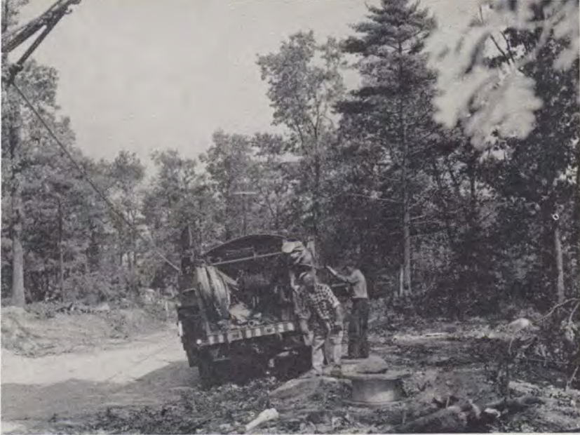
Surrounded by rubble and debris a New York crew works at Farm Hill Lane, Hingham.
