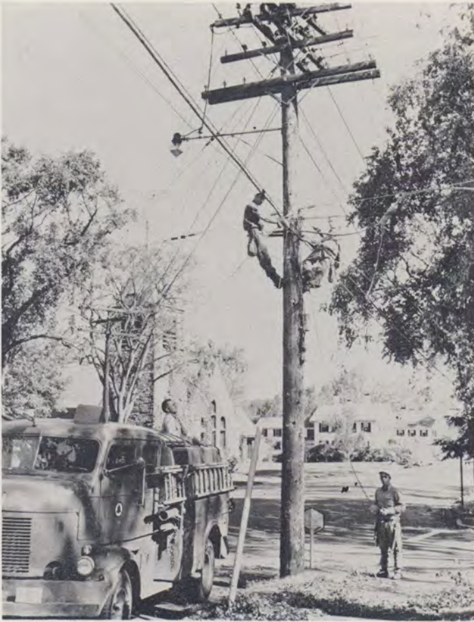
LEFT: Intra-company cooperation demonstrated as the crew from Vermont restores lines at Central and School Streets, Andover, Mass.: Robert McAvoy, D. Beattie, R. Callahan, P. Gale. BELOW: Two New Jersey Installers lend a helping hand to Frank Farrell, Nashua C.O. repairman, in the Derry, N. H., exchange.
